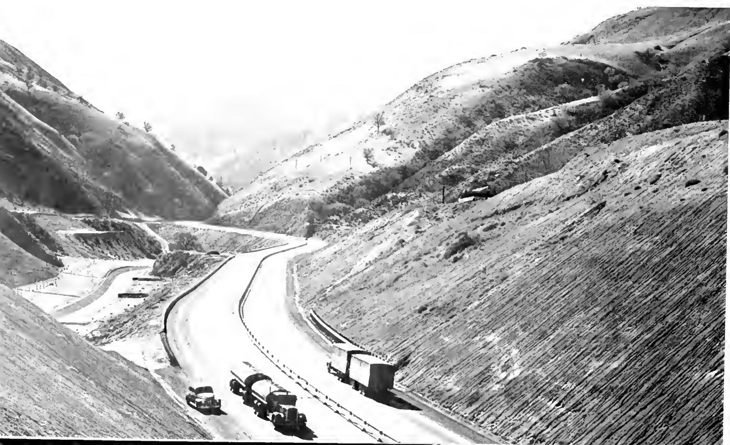
Section of new 4-lane divided highway in Grapevine Canyon, showing metal plate road divider and concrete flume for creek at left.
